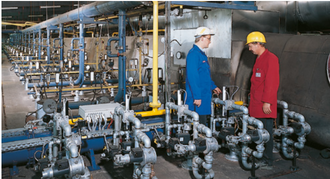
Gas train in a brickworks
