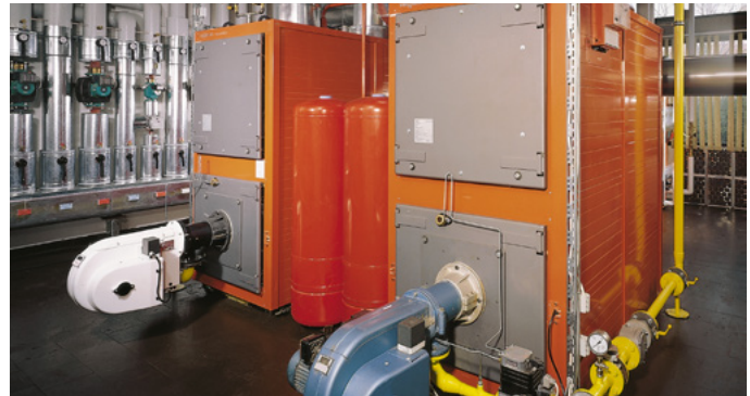
Gas inlet pressure monitoring on high-performance boilers
