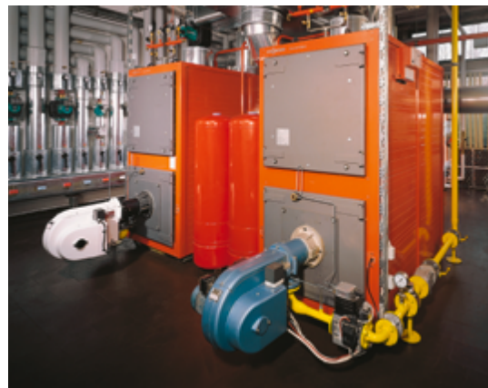
Gas inlet pressure monitoring on high-performance boilers
